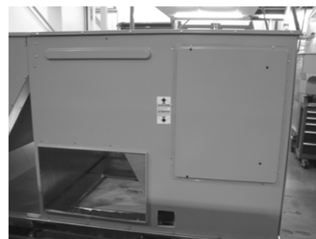
Figure 16: Side Duct Connection
